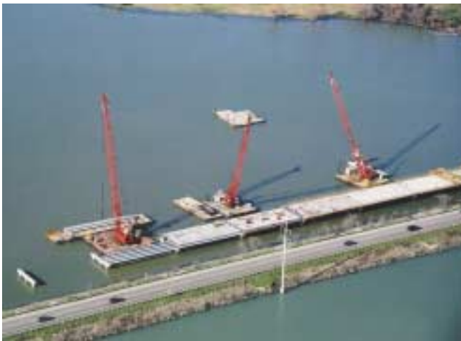
After the drill shafts are drilled, poured with concrete, and caps are formed and poured, the deck construction begins.
