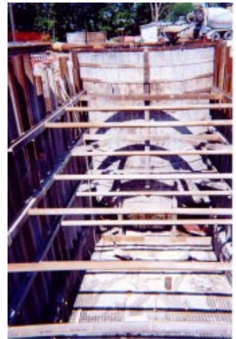
This photo shows ground support for connecting tunnel/spillway excavation. The south side of the rib and lag shaft have been exposed and the rock removed. The excavation bracing is holding the shaft in place.
