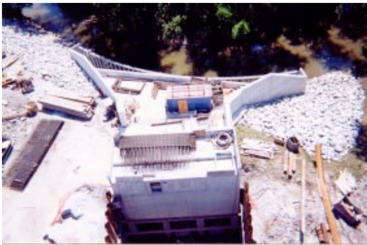
Intake Structure at Thorn Creek houses three 12x12 foot sluice gates and the associated control equipment.
