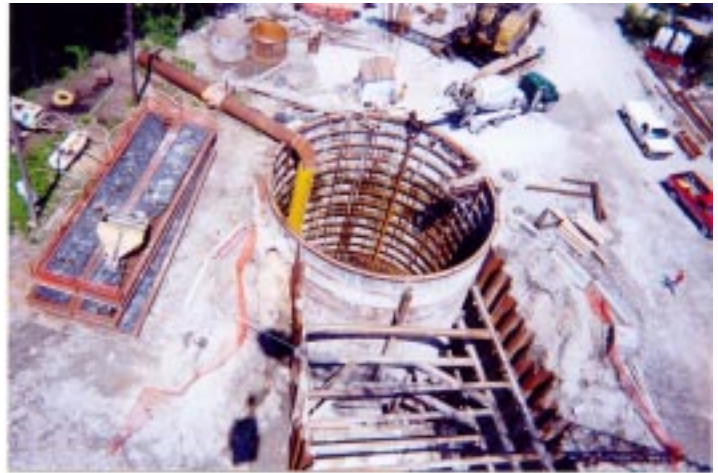
Main drop shaft where the floodwater will drop into the deaeration chamber on the way to the reservoir. One of many concrete pours is underway.
