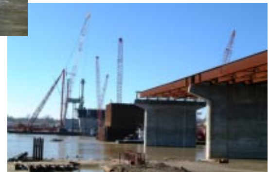
At right are Piers 2, 3, 4, 5, 6 from the Illinois bank. Construction in March shows Pier 2 in the distance.
