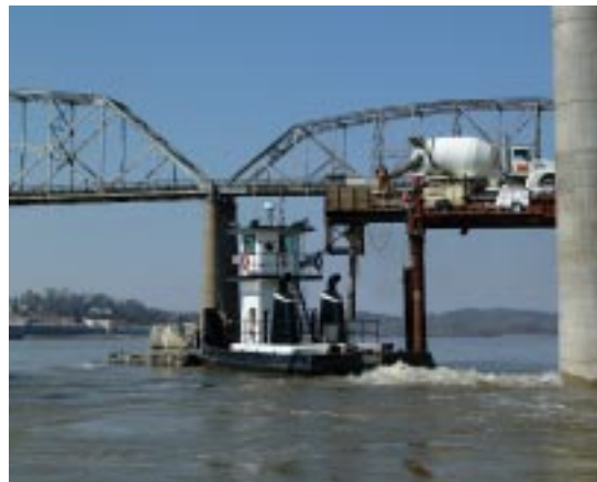
Above, the Potomac pulls away from the trestle after filling 2 laydown buckets with concrete during a Pier 3 tower leg pour.
