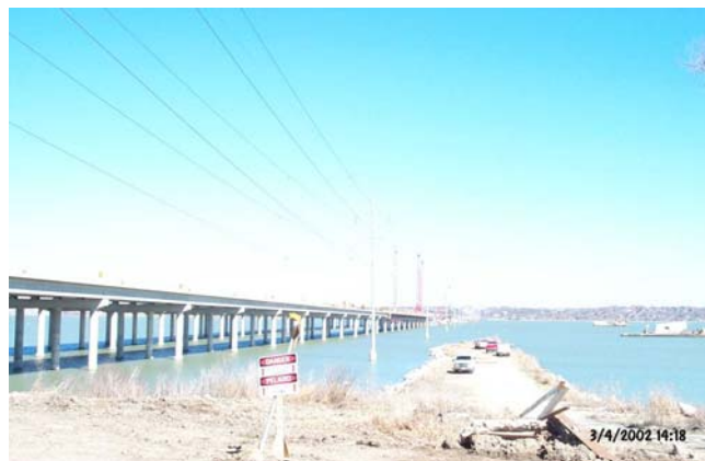
Eastbound bridge under construction. View shows powerline interference requiring use of trestle.
